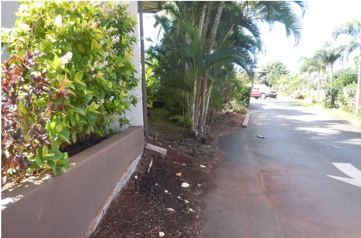
This downspout at Hale Royale discharges roof runoff onto exposed soil, which then is eroded and carried into the driveway and out into the street.
